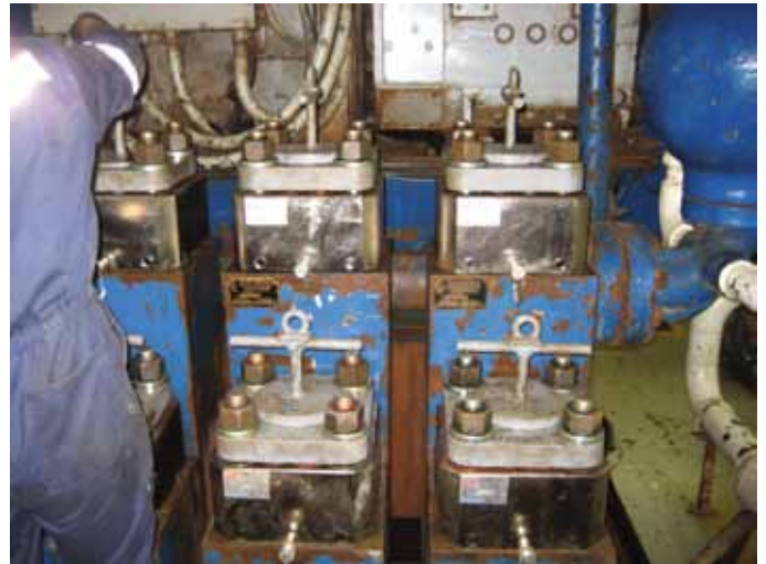
Mud pomp (foto SodM)
