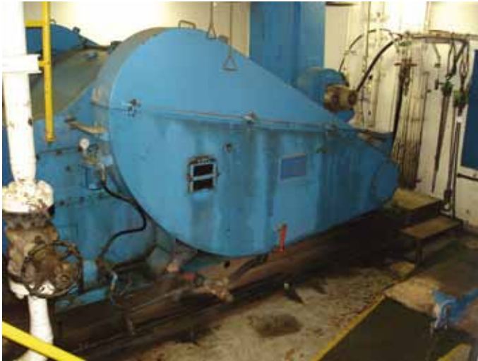
Mud pomp (foto SodM)
