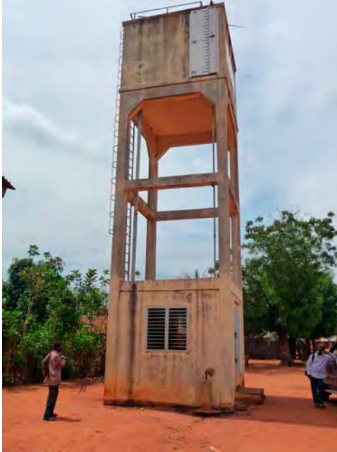
Water tower small piped water supply system
