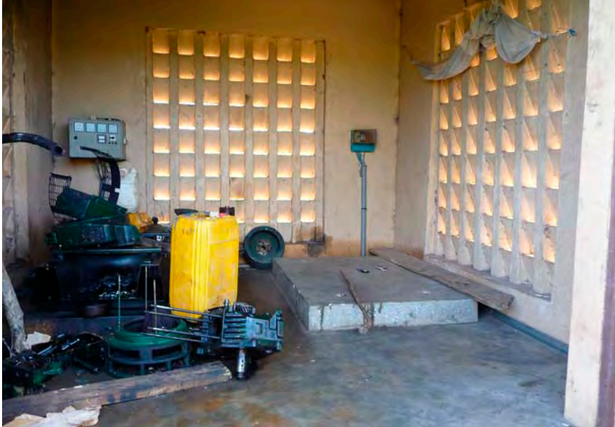
Collines, broken small piped water supply system
