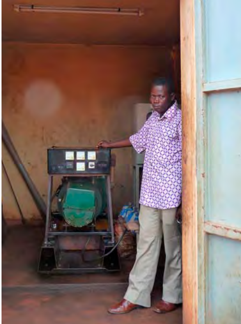
Exploitant small piped water supply system
