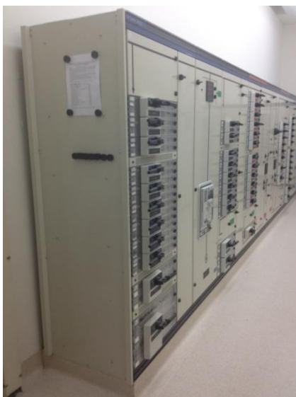
Figure 7-5: Electrical cabinets in the low voltage room at ground level
