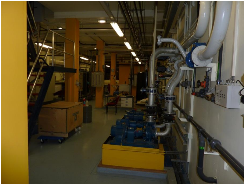
Figure 7-3: Water treatment room in the basement
