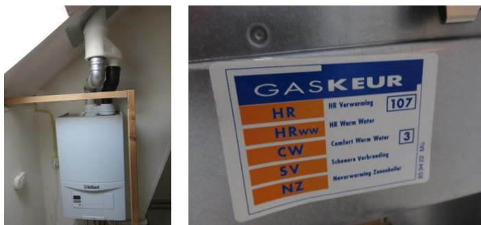
Figuur 43: HR-107 ketel woning 127
