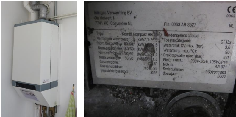
Figuur 61: HR-107 ketel woning 176
