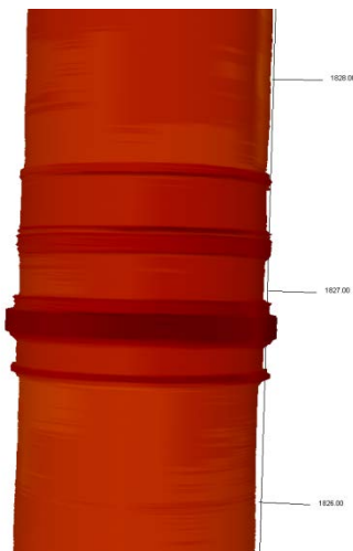
Figure 7 – 3D-calliper image of potentially undertorqued casing joint in TUB 10 at 1827 mAHbdf. The section shown is about 2.5 m long, the segment with a slight diameter increase is about 15 cm long.
