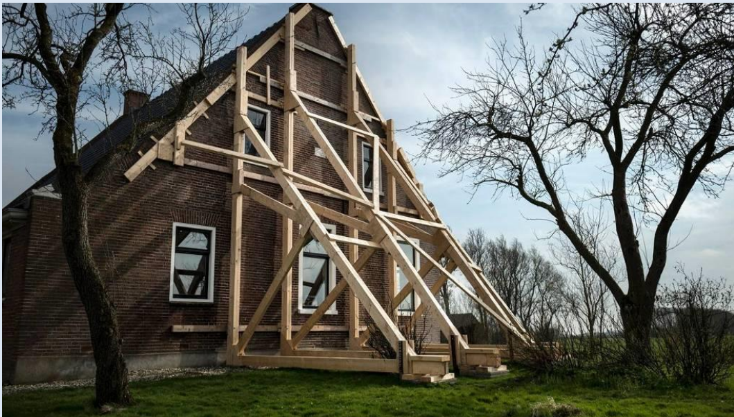
Schade door aardgaswinning [57]
