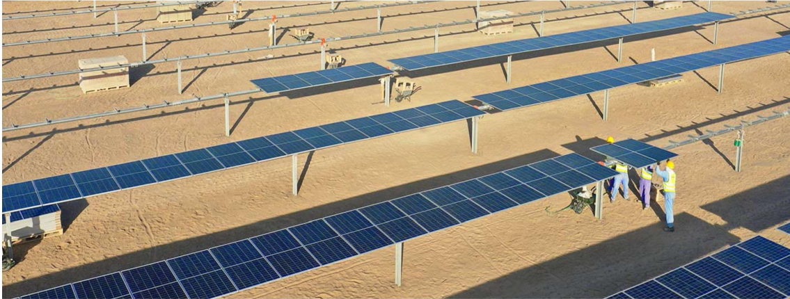
Workers installing one of 1.4 million solar panels that make up the Ibra II 500-megawatt solar photovoltaic independent solar power plant, the largest utility-scale solar park in Oman. Photo © AIIB 2021
