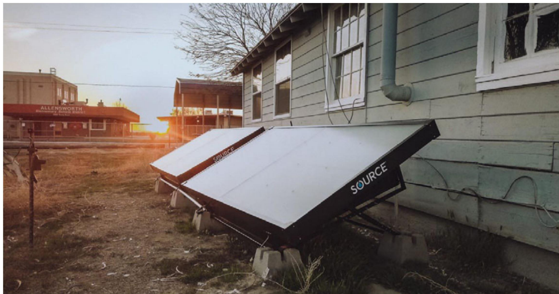
Solar panels, part of the water-from-air harvesting technology, a project in Timor-Leste funded by Lightsmith, a financing partner of AIIB Photo © SOURCE Global, PBC 2021
