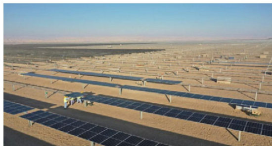
Workers installing one of 1.4 million solar panels that make up the Ibra II 500-megawatt solar photovoltaic independent solar power plant, the largest utility-scale solar park in Oman. Photo © AIIB 2021
