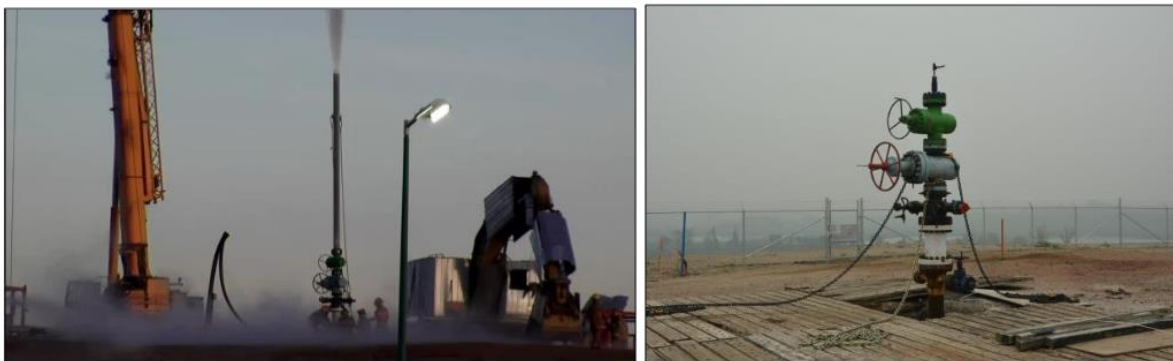
Figure 38. The first photo (right) was taken right after the fire had been extinguished and the new wellhead lowered in to place. A temporary vent stack has been attached to the top of the wellhead. The second photo is from June 2015 and more clearly shows the new wellhead chained in place. Acknowledgment: Dave Burdeniuk.
