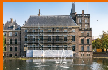
An extensive maintenance project, the Dutch historical Binnenhof is now being renovated to modernise its systems, welcome more visitors in the future and become more accessible for people with a disability.
